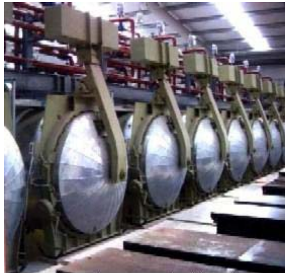
Autoclaves with counter-weighted doors shut Advanced Technology in civil engineering
