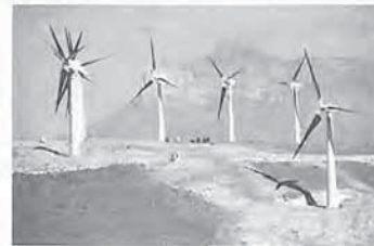
FIGURE 1.20 Efficient wind power generation in west Texas. (Used with permission of DOE/NREL. Credit: Lower Colorado River Authority.)
