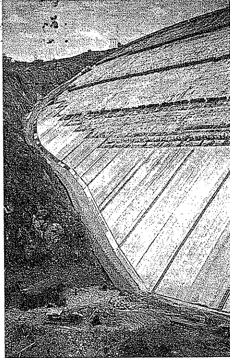
Figure 9.39. Concrete face sealing. Photograph shows the starter slabs from the plinth to the horizontal contraction joint and the shotcrete cover on the transition layer.
