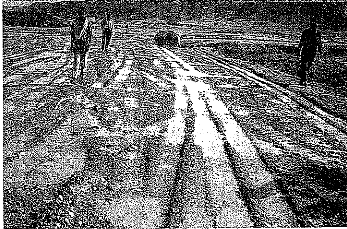
Figure 9.21. Placing of sand-gravel with addition of water. The amount of water is excessive; the compaction is not fully effective (courtesy of LI).
